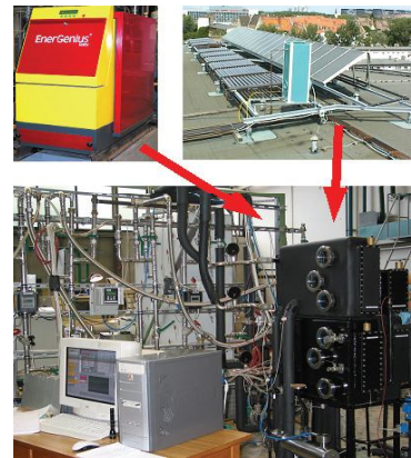
Fig. 1. Absorption chiller under test at TU Berlin, operated by cogeneration engine (upper left picture) or solar collectors (upper right picture).
