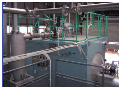
Figure 2. Commercial plant of the hydrothermal treatment.
